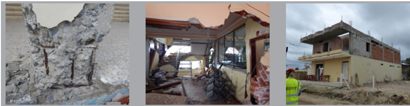
Evidence of poor construction practice and lack of earthquake safety measures associated to non-structural elements
