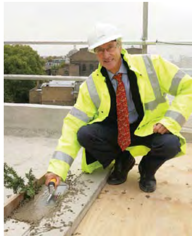
Sir Richard lays the final piece of concrete in Imperial's new student accommodation
