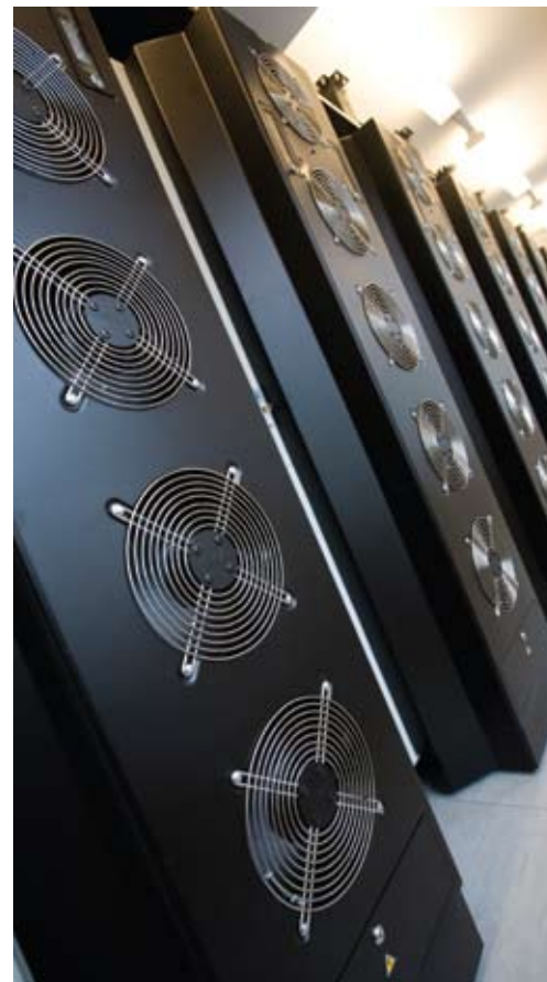
The HPC service, housed in the ICT Data Centre, has proved very popular with users from all faculties and Tanaka Business School since the service went live in 2006
