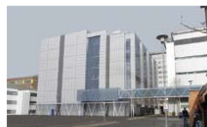
[Top] Construction company Bovis Lend Lease have started work on the foundations for the new L block development. [Bottom] Artist's impression of the new L block, due for occupation in 2012.
