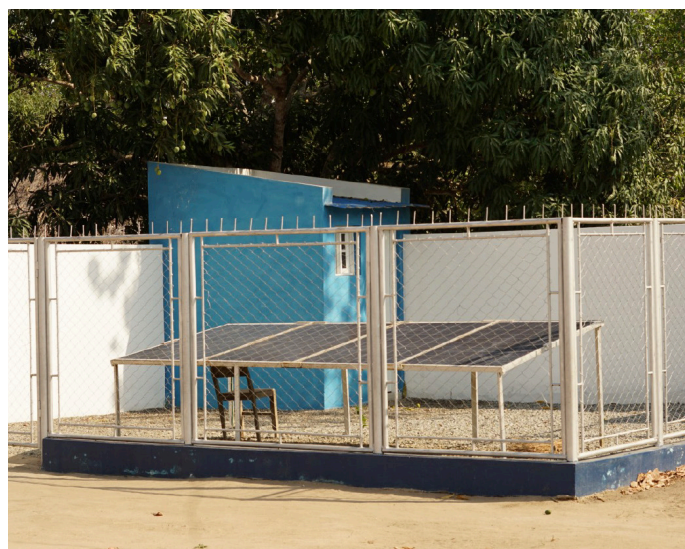
Solar panels that are part of the water supply system in Mossuril, use a renewable source of energy to pump water to the community.
