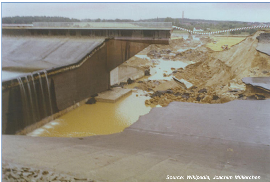
dam breach at road tunnel after flooding of a new canal section
