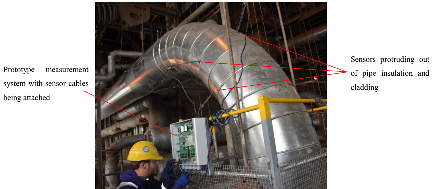
Figure 7.3: Photograph showing sensors and measurement system installed at West Burton power station.
