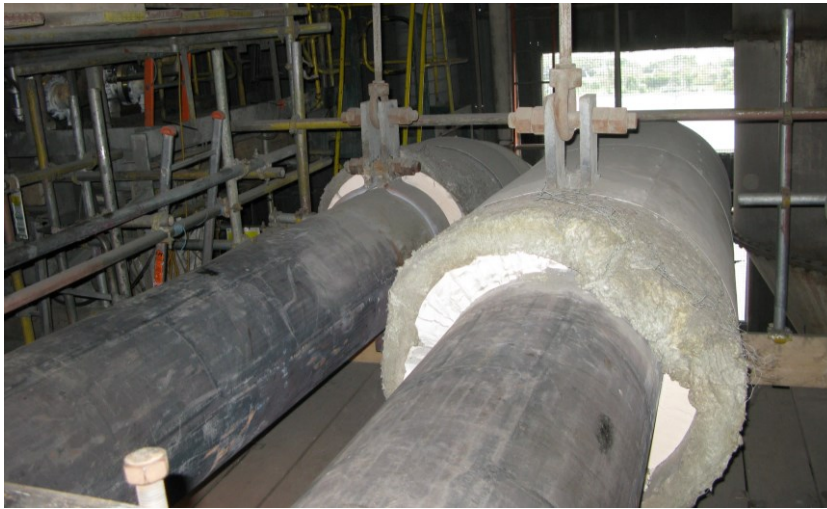
Figure 1.4: Photograph of CMV hot reheat pipes. Two pipes are shown during an outage. Hangers to suspend the pipes are shown in addition to thermal insulation which covers the pipes during normal operation.
