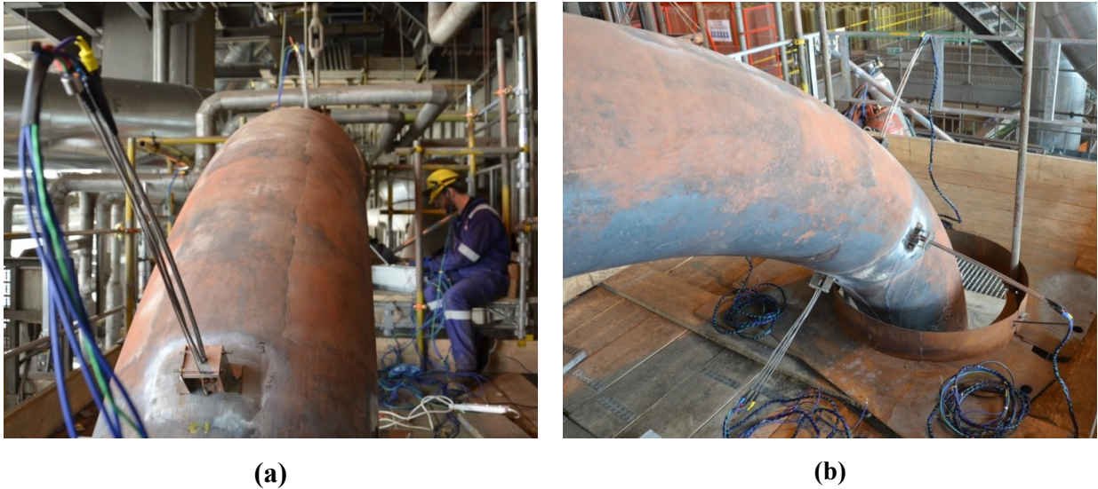
Figure 7.2: Photographs of potential drop sensors installed at West Burton power station.
