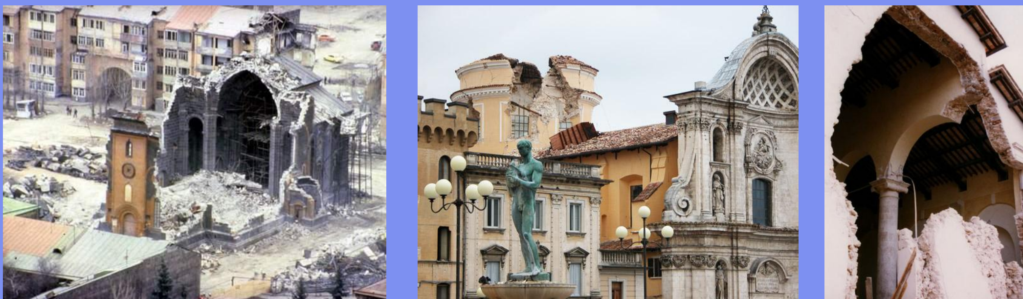
Figure 1: Damage and collapse of historical masonry structures
